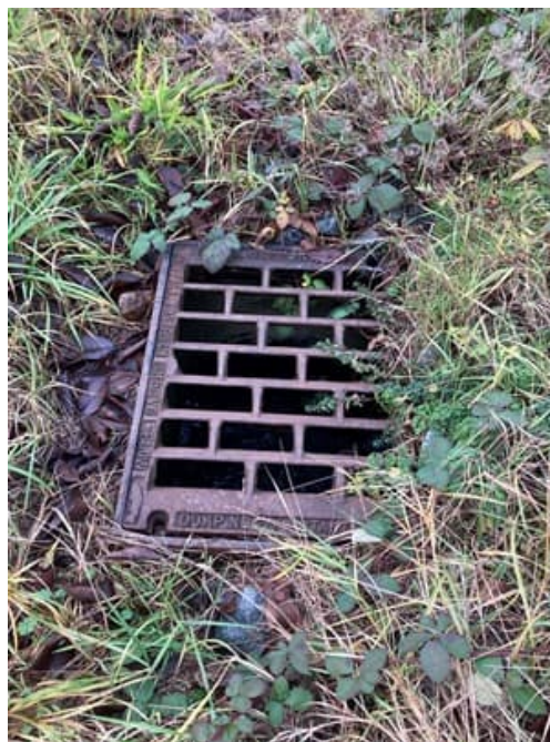
Picture 6: ROW CB next to driveway of 2825 W. Mercer Way (vacant lot) Water continues flowing west
