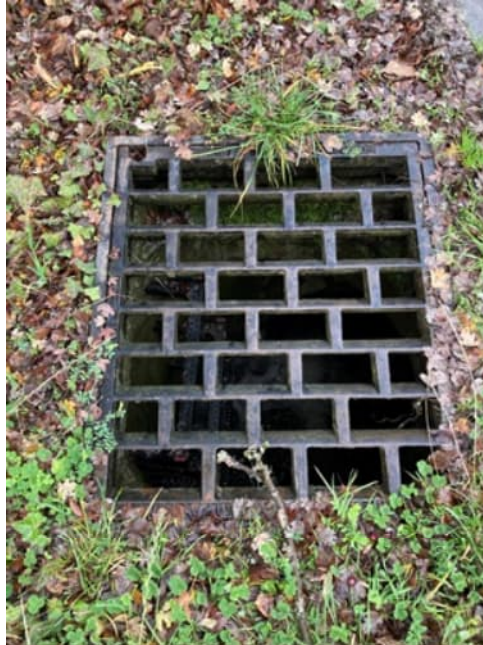
Picture 5: CB at the SW corner of 63 rd Ave SE and SE 28 th St Heading west
