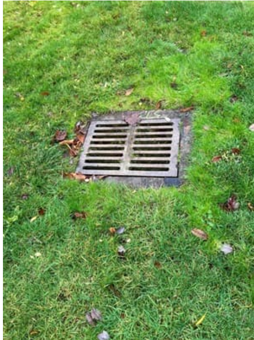
Picture 11: ROW on the north side of 2800 60 th Avenue SE, looking west
